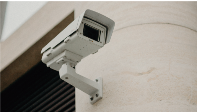
Closed Circuit Television (CCTV)
